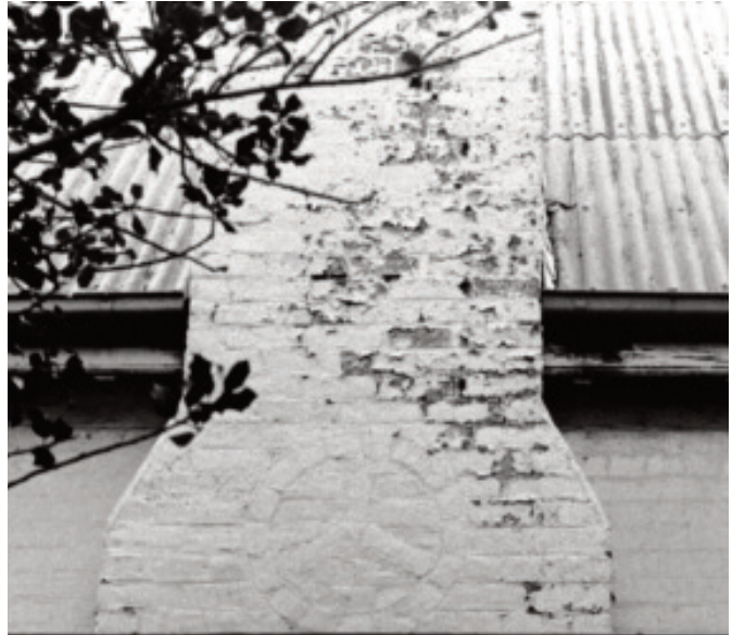
Detail of inlaid brickwork symbol in chimney, Springside School. Source; John Kich, 1979.
